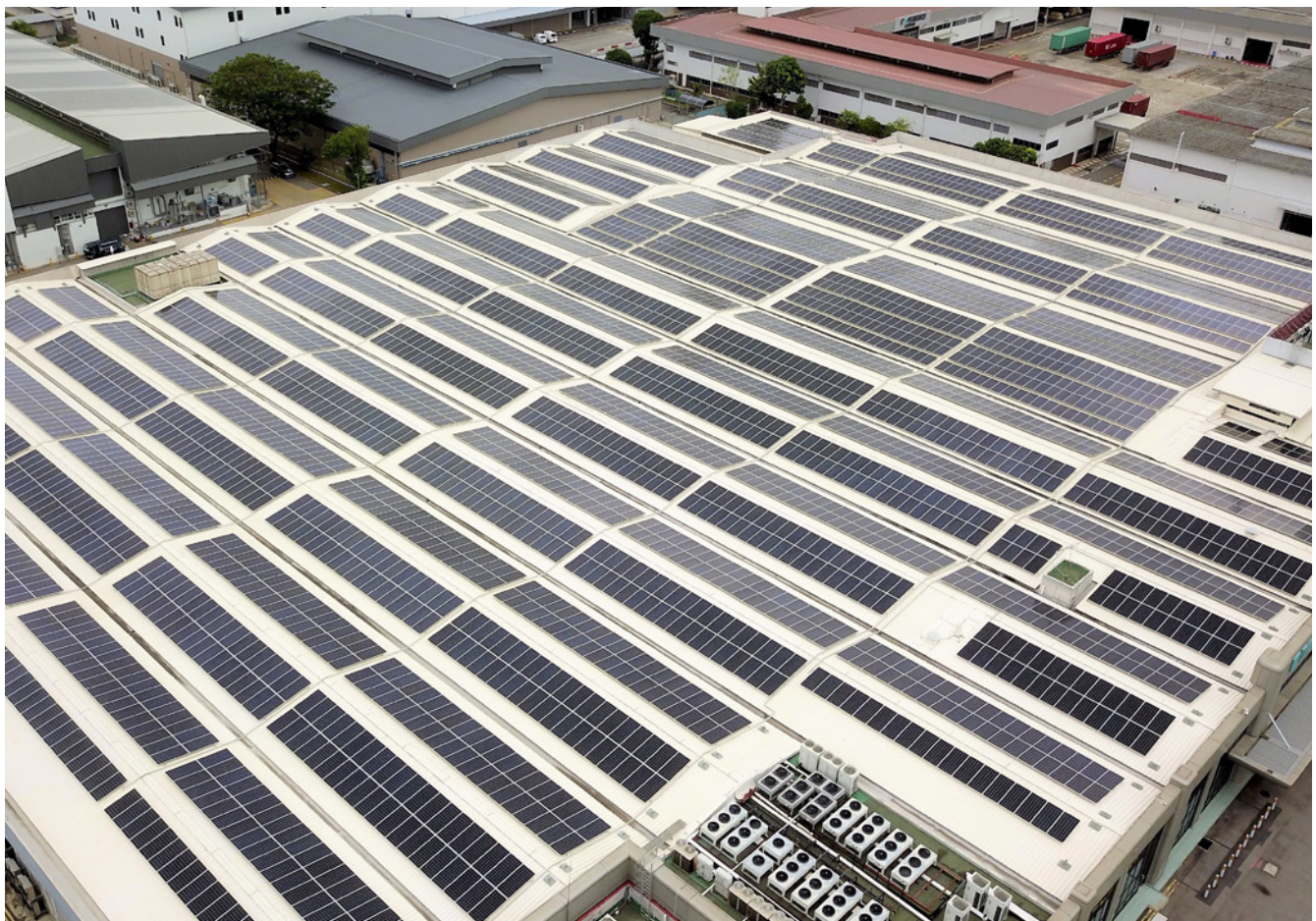
Solar panels on the rooftop of NCS Bedok Data Centre
