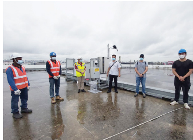
WSH team and contractors installed new remote monitoring system on a rooftop which houses our 5G equipment
